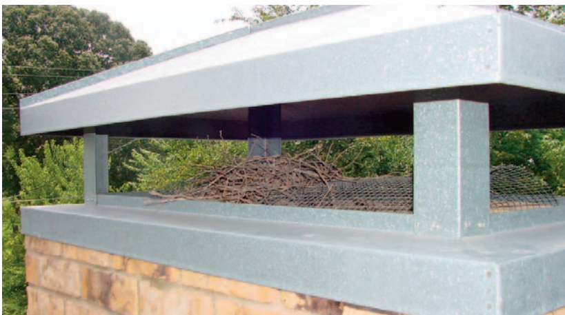
Figure 1. Close up view of the position of a Northern Mockingbird nest beneath the metal rain guard of a chimney (photo courtesy of Timothy J. Bister).
