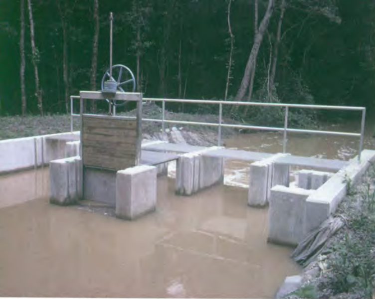
Water control structure USFWS
