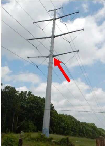
Figure 2. A metal mono pole with tubular cross-arms where American Kestrels are nesting along the Burtonsville to Takoma transmission line in northwestern Prince George’s County, Maryland. Location of the kestrel access at the base of the cross-arm.
